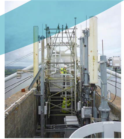
Scaffolding access at the top of Saltash Tower to allow remedial works to take place.
